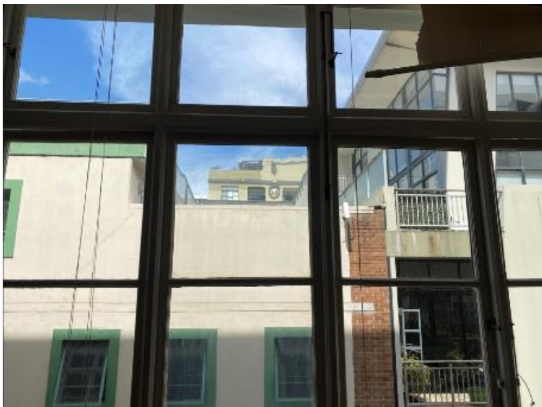
Figure 42: Internal view of Unit 43, looking east towards Hands Lane. Image supplied by resident
